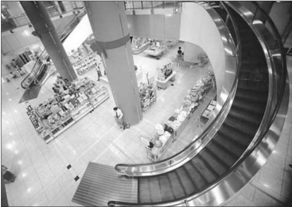
FIGURE 11.14 A spiral escalator effectively used in the Yamako Department Store in Kofu, Japan. (Courtesy Mitsubishi Electric Corporation)
